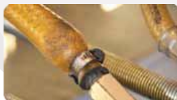
An illustrative example of a leaking coupling with hose clamp.
